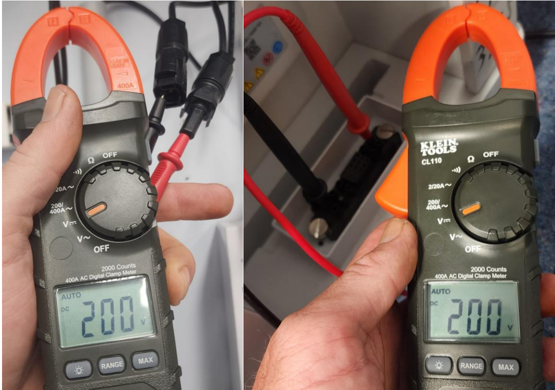
Photos of battery voltages at the base and at the inverter
