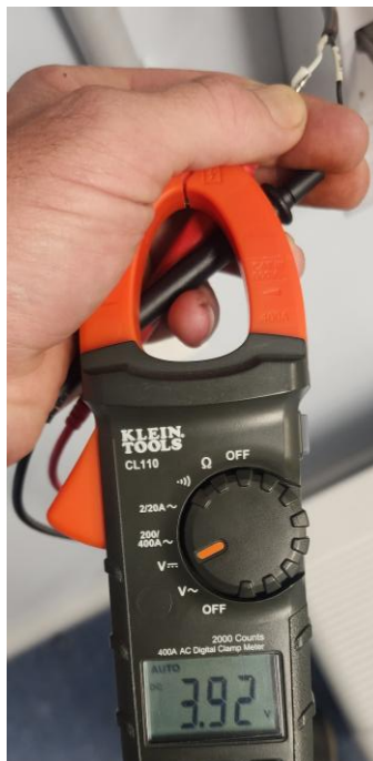
A photo of the RS485 cable at the inverter end showing that the signal from the meter is getting to the inverter end
