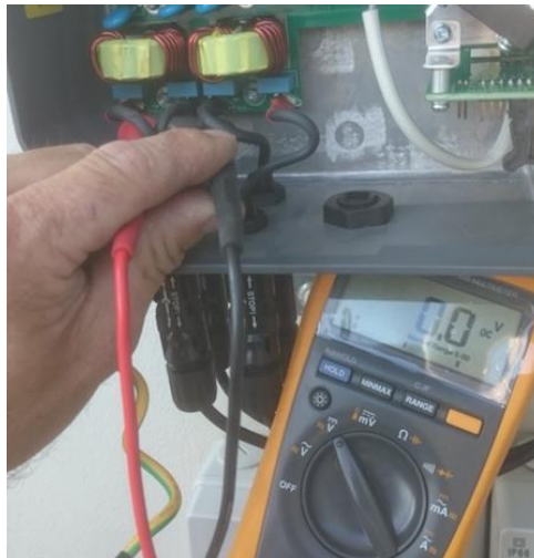
Figure 4 No Internal DC Voltage
