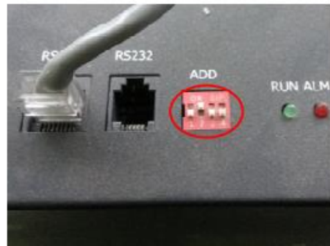
Figure 3: Master battery address
