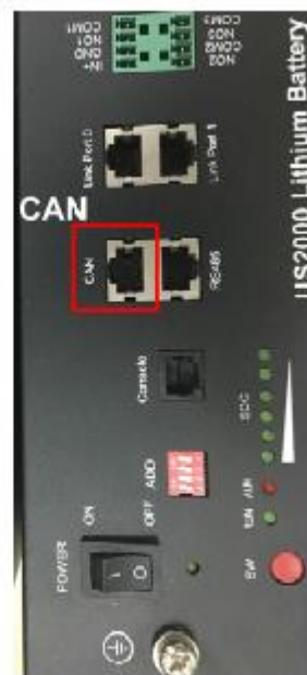
Figure 11: CAN port on the battery
